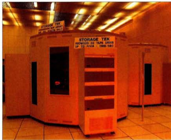
One of CERN's StorageTek tape silos used in the ALICE data challenge.
